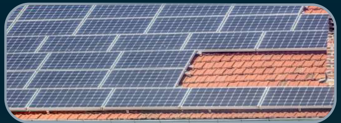
Distributed solar PV
